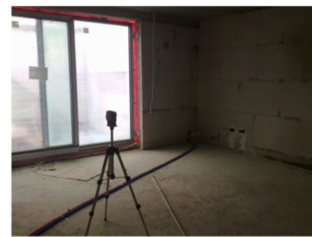
First step is to level the laser with the mark on the wall
